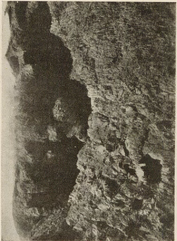
Fig. 2.—Cavity between the back of wall and the rock.
